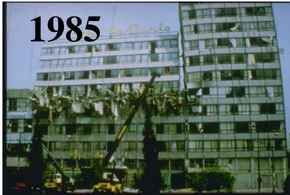
Earthquake Damage in Mexico City, Mexico, September 19, 1985 - resonance
