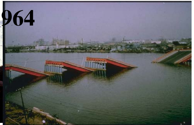
Showa Bridge after 1964 Niigata earthquake
